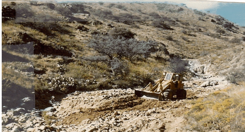
TWO SECTIONS OF THE ROAD WASHED OUT AT THIS POINT KM 14
